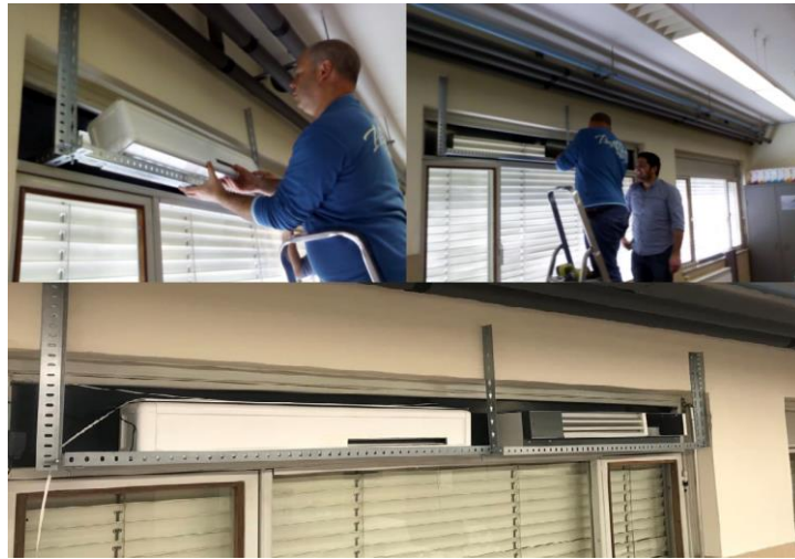
Figure 4.3 – Installation of the Smart Window ventilator boxes prototypes at the I2L office.
