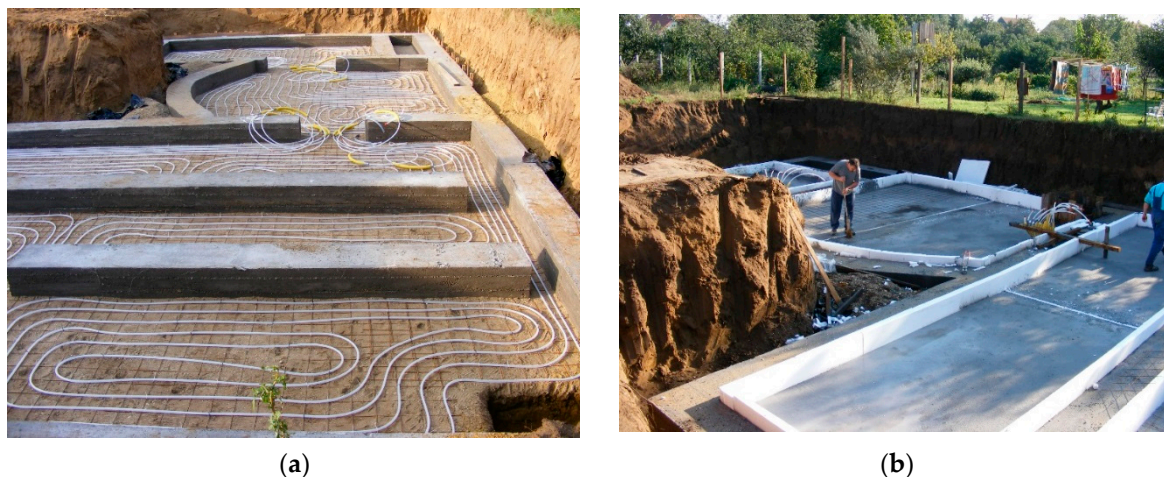
Figure 4. Hydronic tubing installation in the ground-floor slab. Courtesy Thamas Barkanyi. (a) Hydronic tubing before concrete pouring; (b) Edge thermal insulation and covered tubing.
