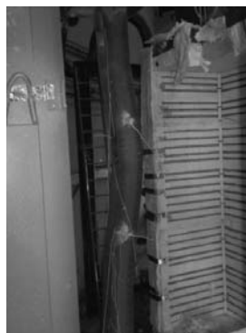
Figure 6: Column E18 after test
