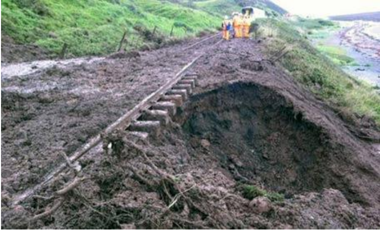
Figure 2-9 Damage to the rail infrastructure in Cumbria, UK, in August 30, 2012 caused by rainfall-triggered landslides. (Network Rail in BBC News (2012)).
