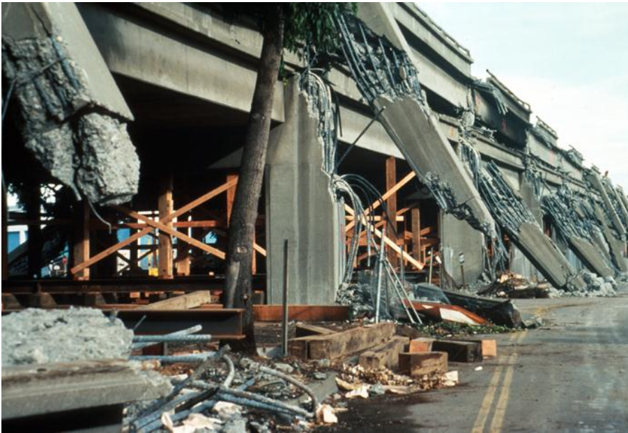
Figure 2-11 Support column failure and collapsed upper deck on the Cypress viaduct, Oakland (USGS 1998f).
