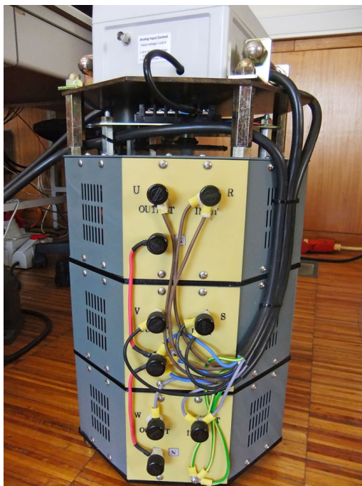
Figure A.1: Autotransformer used to supply the PMSG drive.
