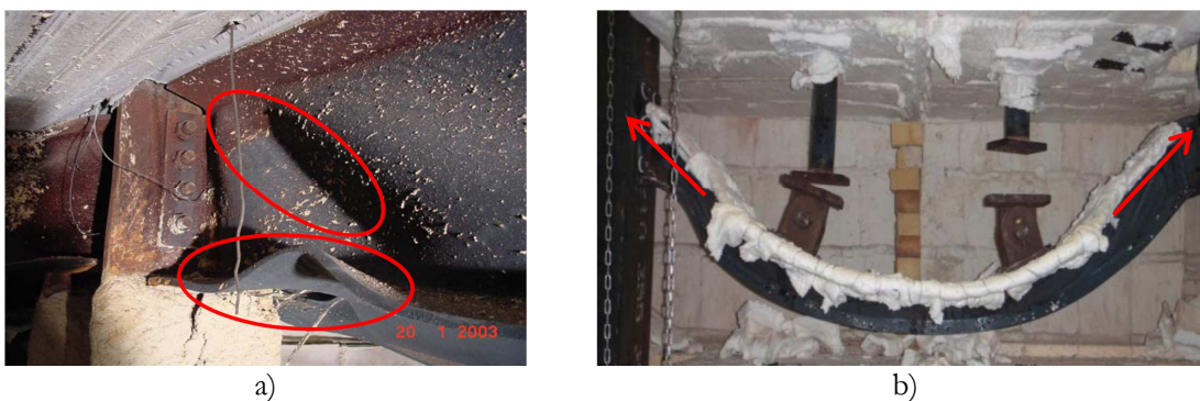
Figure 1.3: a) Local buckling of beam web in shear and beam flange in compression (Santiago, 2008); b) Catenary actions (Simões da Silva et al. , 2013)
