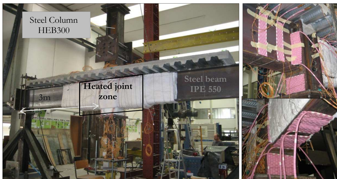
Figure 3.13: Heated connection zone using Ceramic Pad Heating elements, thermally insulated by rock-wool of density 128 kg/m 3 (tests 2 to 6)
