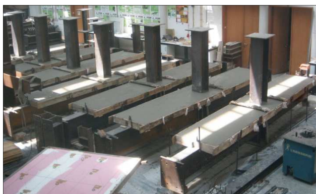
Figure 3.6: Specimens after the concreting of the composite slabs, at the floor level
