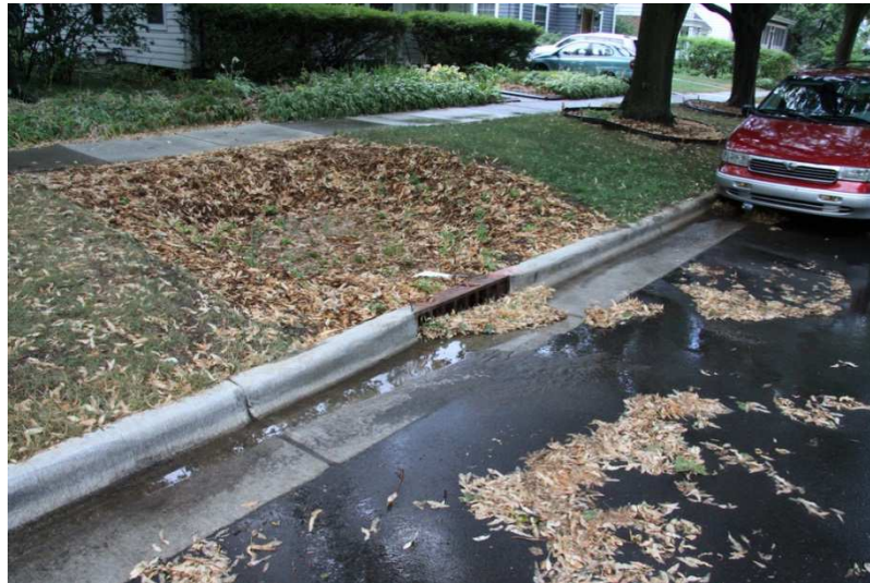
Figure 2.9 – Clogged inlet in Lake Wingra, USA (wingrawatershed@, 2012)
