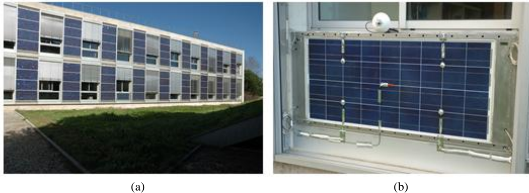
Figure 1. (a) Prototype installed on the SolarXXI main façade; (b) BIPV-PCM system.
