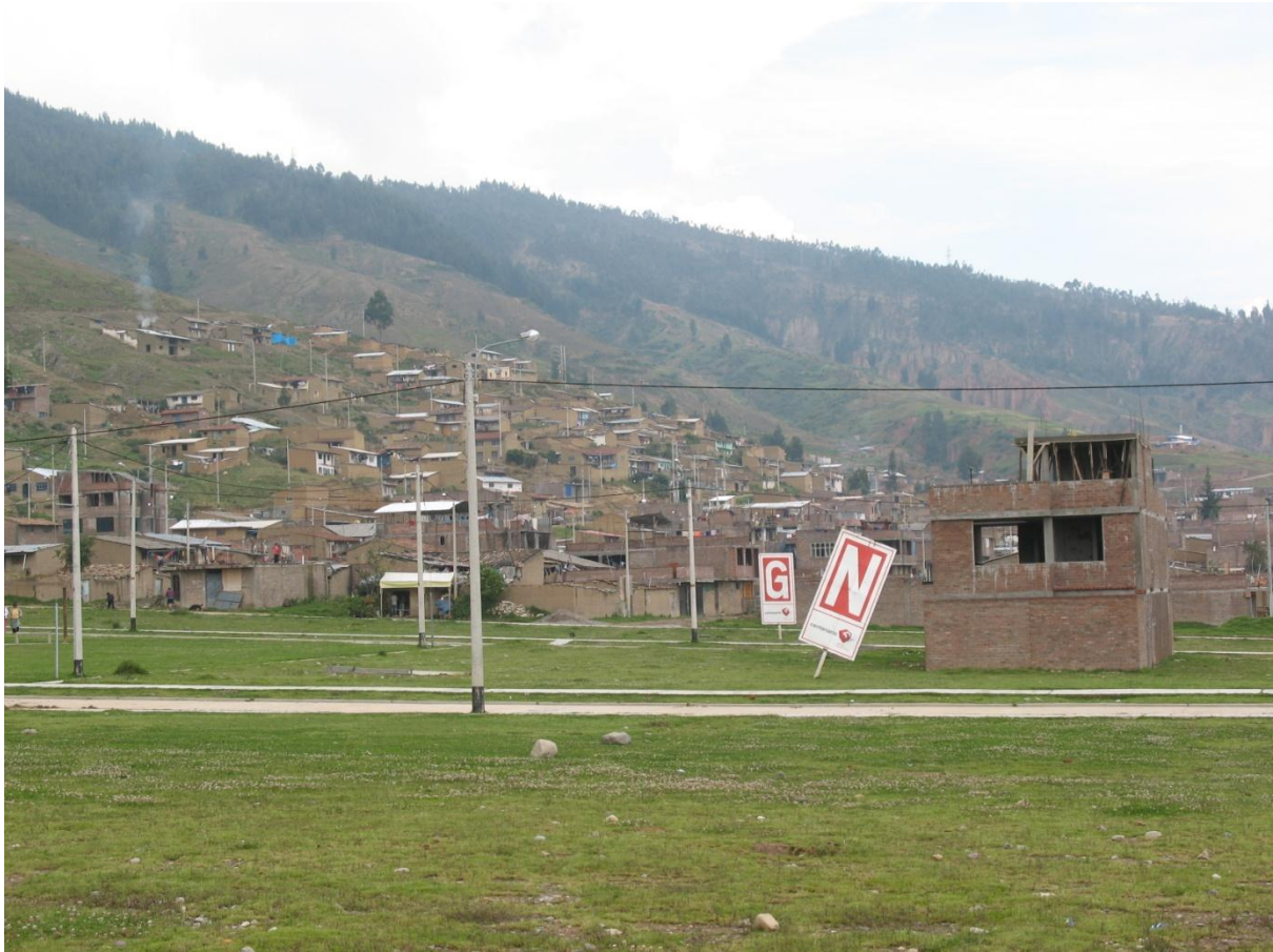
Gated community Alto la Merced under construction. In the background is the informal settlement Santa Isabel, Huancayo 2012. Photo by the author.
