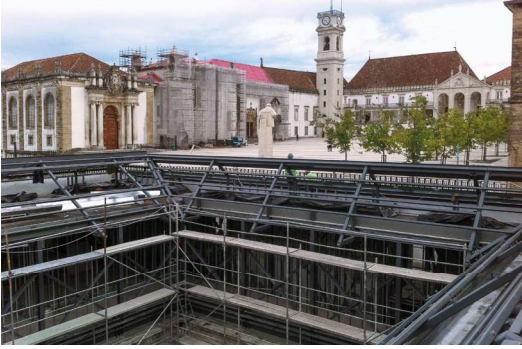
Figure 5. Photo of the steel structure with Courtyard of the University of Coimbra in the background, October 2015.
