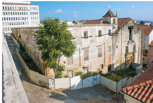
Figure 1. View of the facade of the College and the Church of the Holy Trinity after the works of consolidation of facades and before rehabilitation of the building.
