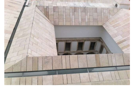
Figure 12. Roof in lioz stone, zone next to the cloister, being visible the continuous traces of zenital illumination
