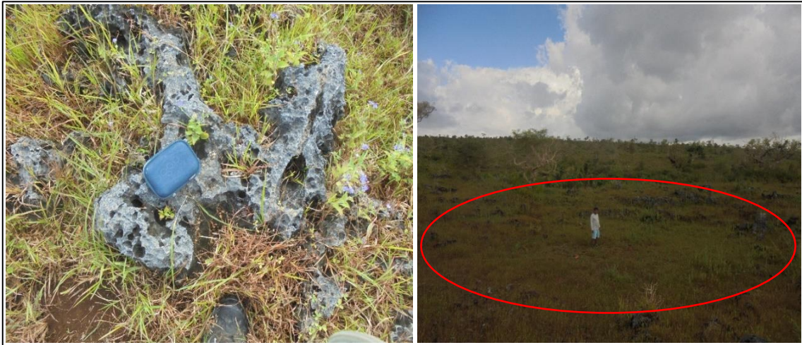
Figure 3. 8 Cavities in the coral-reef limestone (left) and sinkhole (right) in the study area
