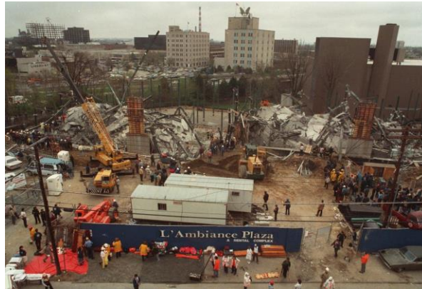
Figure 1-3 L'Ambiance Plaza total collapse (CARTER, 2018)
