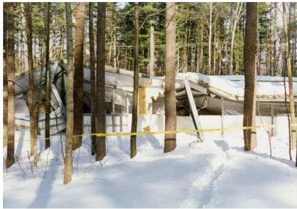
Figure 1-5 Jackson Landing Skating Rink collapse (Technology, 2007)
