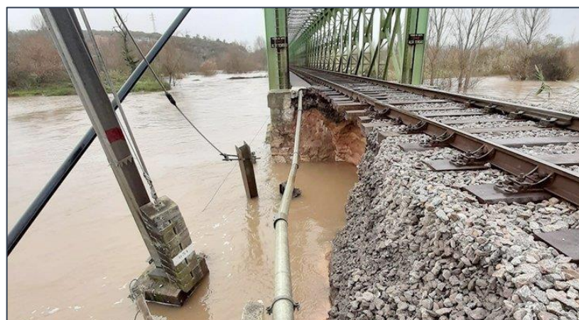
Figure 3.20 – Damaged slope located between Ameal and Alfarelos (IP, 2020b)
