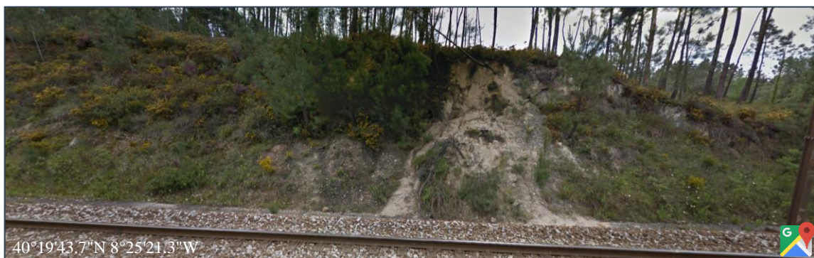
Figure 3.24 – Evidence of slope instability – piles of soil have slid (Google Maps)
