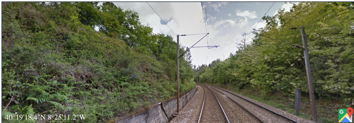
Figure 3.25 – Cracked retaining wall (Google Maps)
