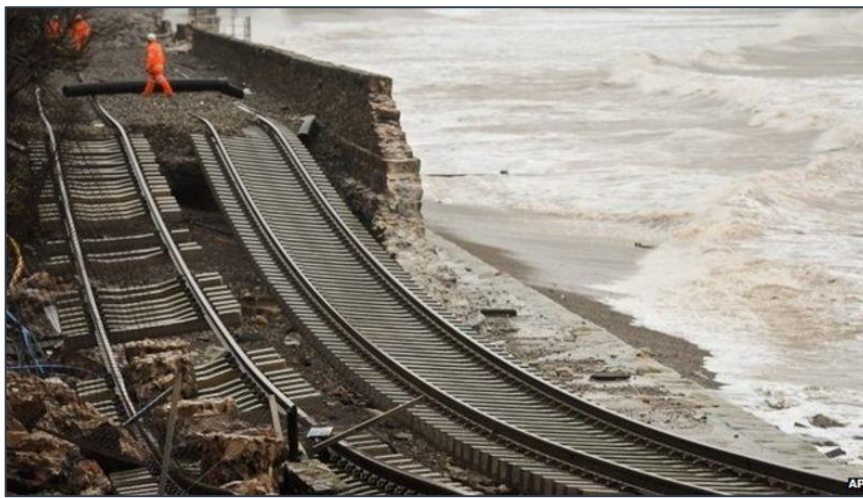
Figure 2.11 – Railway incident caused by a storm surge, UK (BBC, 2014)
