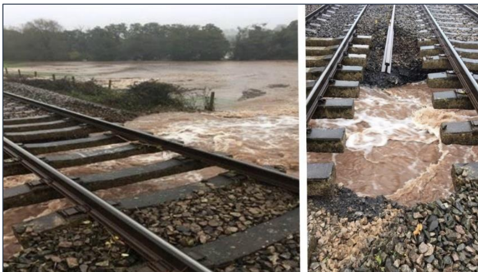
Figure 2.8 – Flood in a railway, UK (BBC, 2019)
