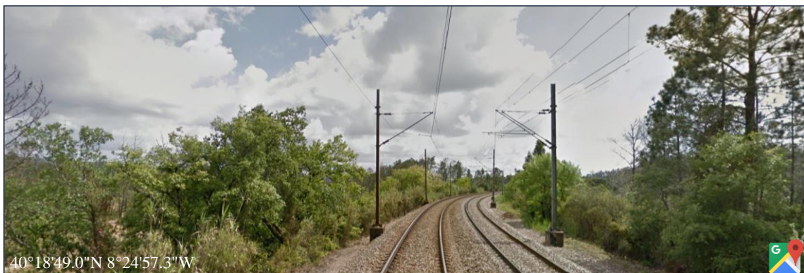
Figure 3.27 – Vegetation on the left may indicate embankment instability (Google Maps)
