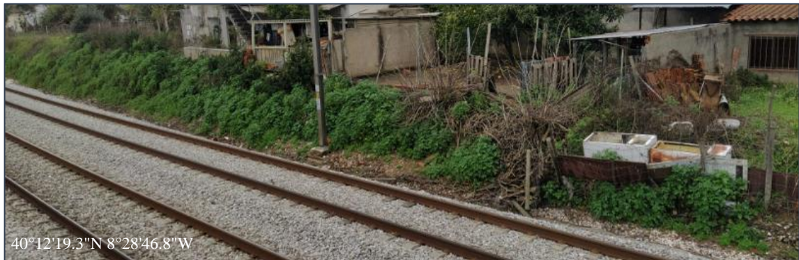
Figure 3.30 – Drainage clogged with debris in Casais
