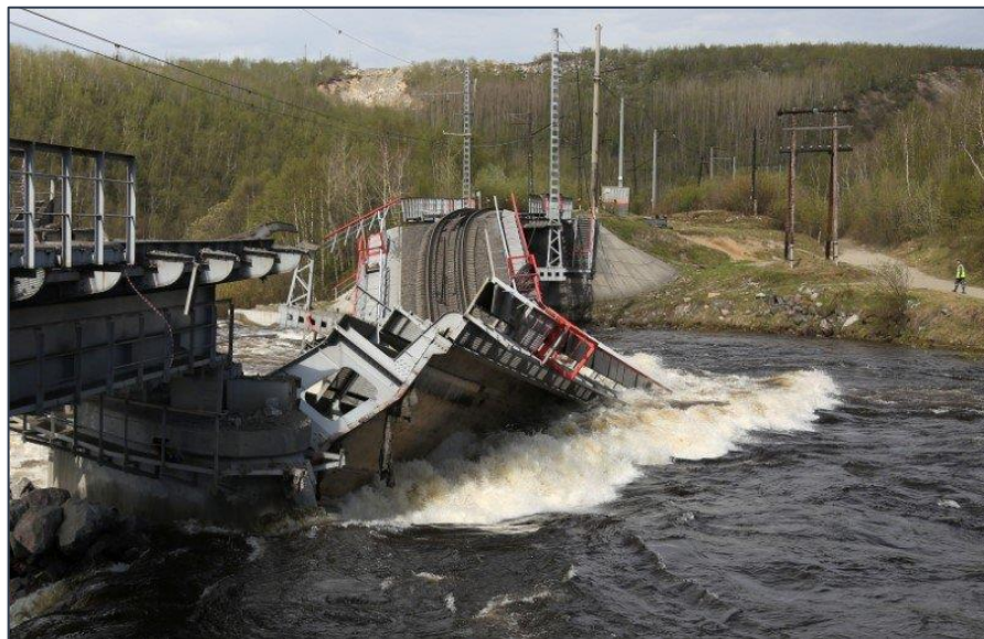
Figure 2.10 – Railway bridge damaged by river flood, Russia (Reuters, 2020)
