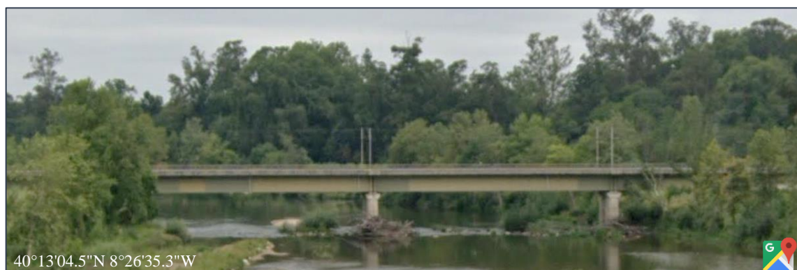
Figure 3.22 – Mondego Novo bridge, Coimbra – piers sustaining debris (Google Maps)
