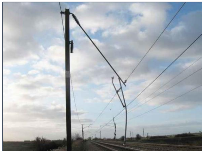
Figure 2.12 – Structure hit by the pantograph, UK (Railways Archive, 2013)
