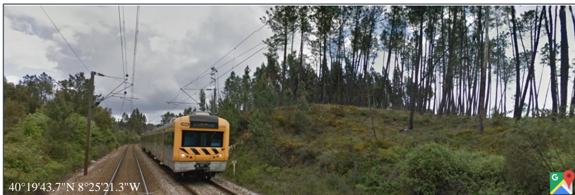
Figure 3.23 – Evidence of slope instability with toppled trees (Google Maps)
