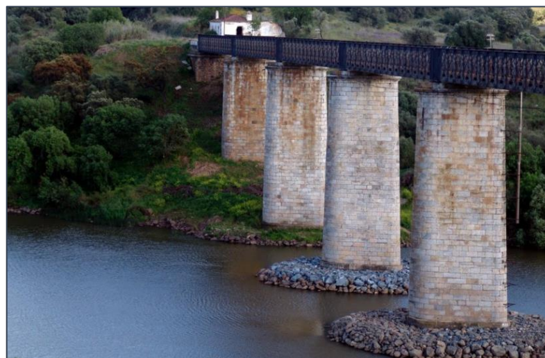
Figure 2.17 – Rip rap technique in a bridge over the Guadiana river, Serpa (Google Maps)
